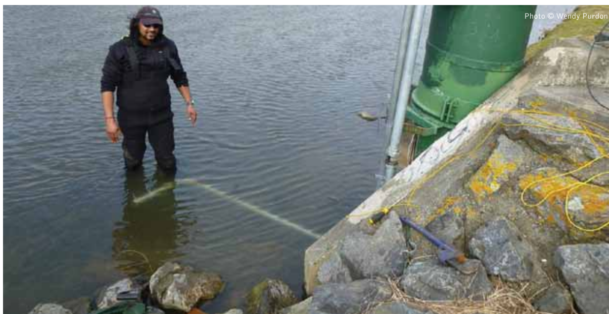
Environmental Monitoring Officer Shyam Morar checking the installation of a continuous turbidity sensor in Porirua Stream, a tributary of Porirua Harbour .
