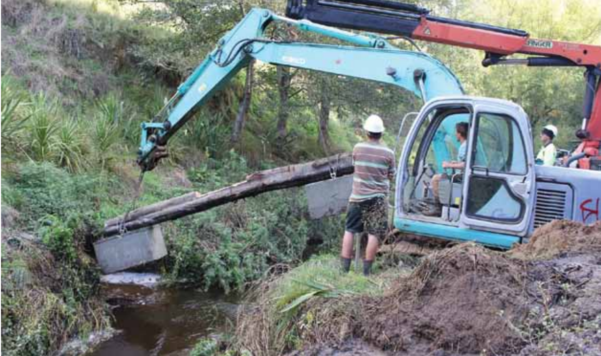
John Carter Constructors installing a woody weir in the Mangakotukutuku Stream, Hamilton..
